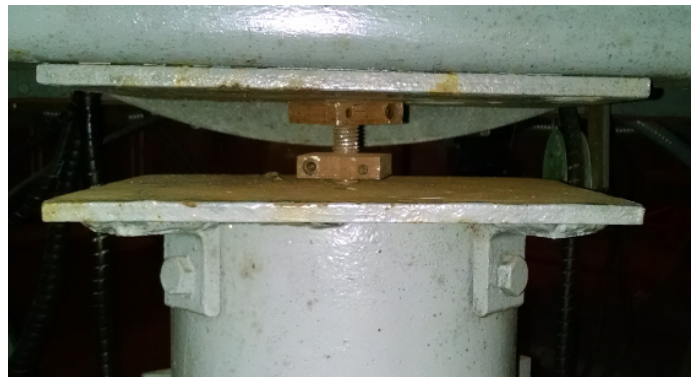
South pier post and plate, and existing solution attaching it to matching plate on mount.
